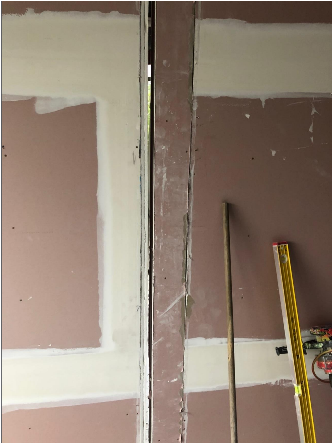
Figure 2: Structural break in bounding wall
