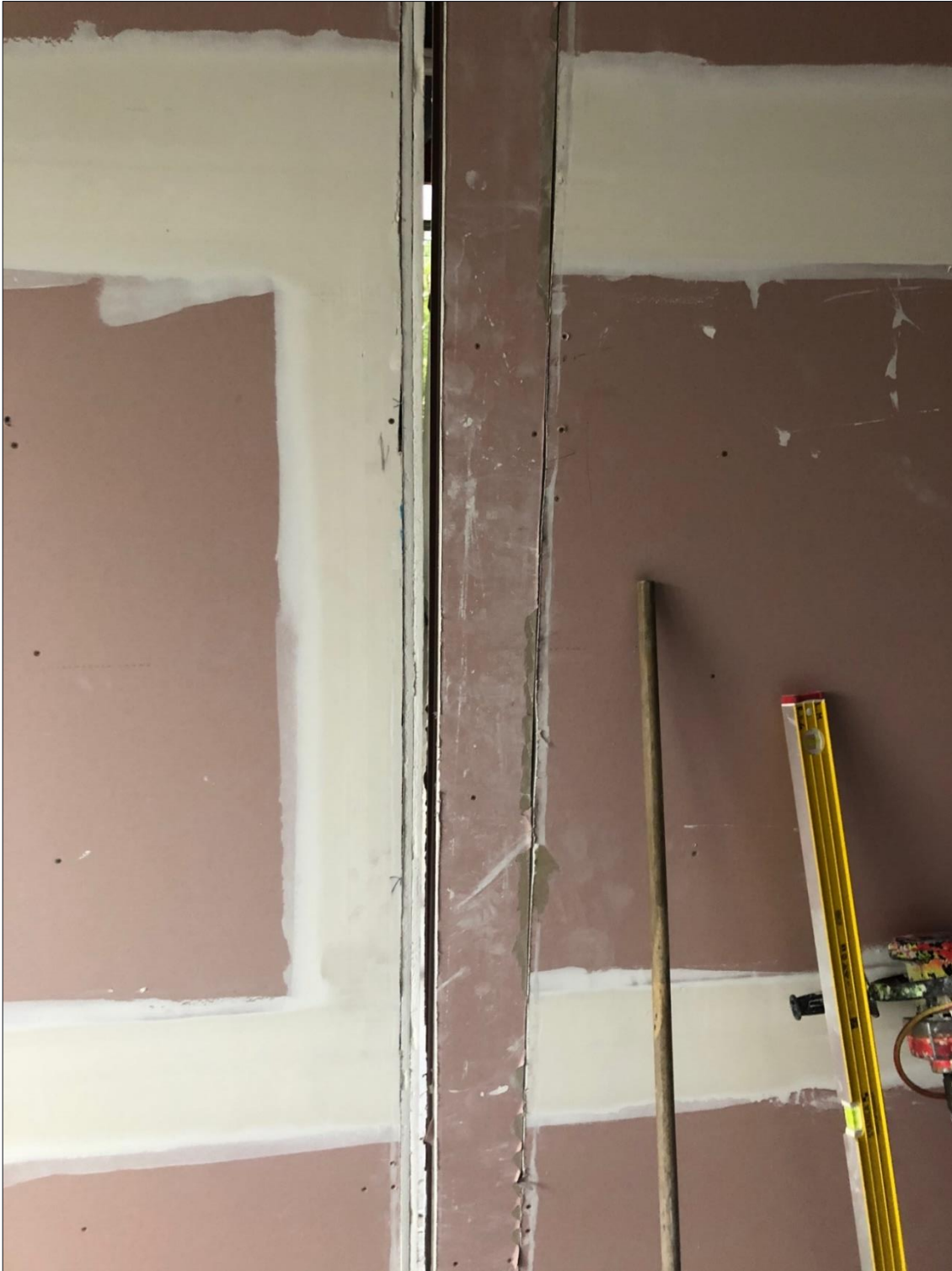
Figure 2: Structural break in bounding wall
